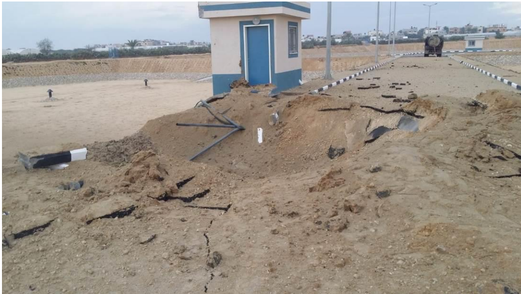
Damages Caused by the Israeli Aerial Strike on the Internal Road of the Infiltration Basins on 11 November 2018
