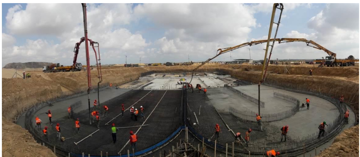
Casting Reinforced Concrete for the Foundation of the Aeration Tank on 20 June 2017
