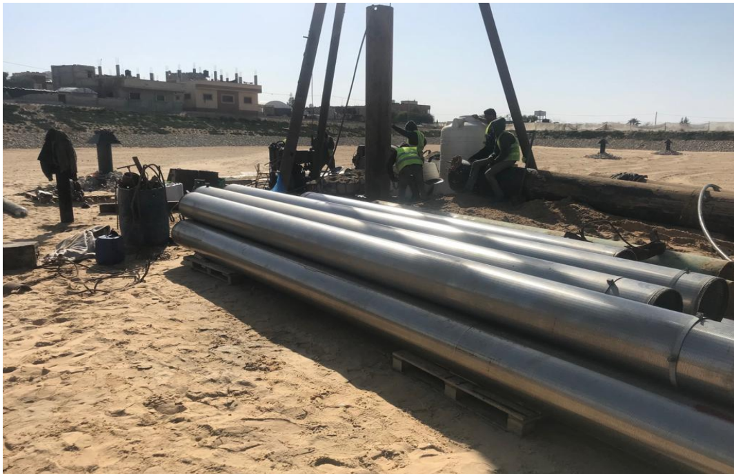
Digging Infiltration Wells and Installing Screens in the Basins from January to March 2019
