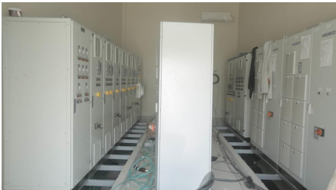
Installed Electrical Panels up to March 2019
