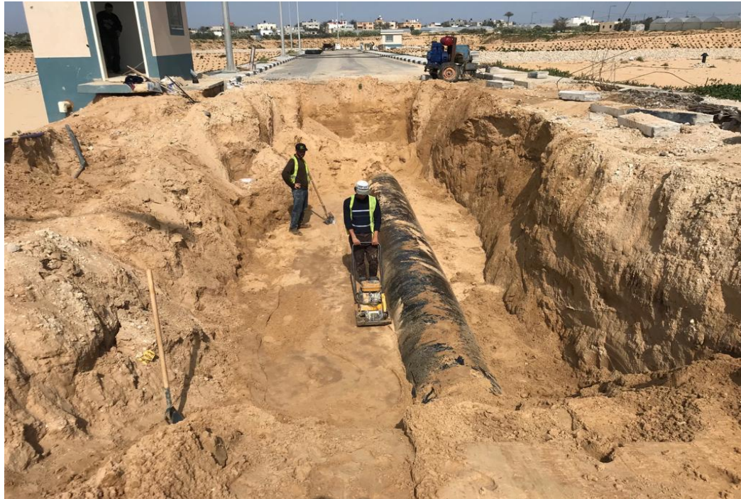
Repairing Damages Caused by the Israeli Aerial Strike in the Infiltration Basins in February and March 2019
