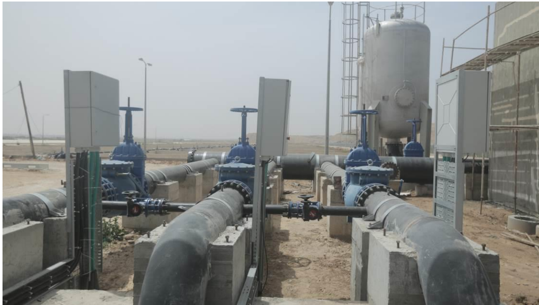
Installed Manifold and Surge Tank for Effluent Pumping Station up to March 2019
